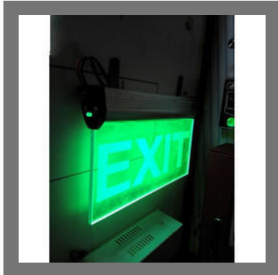
Emergency Exit Light Signage
